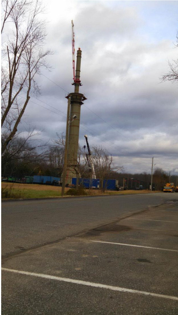
PHOTO ABOVE: Dec. 10, 2014. Early days of water tower construction. Continued on Page 08
